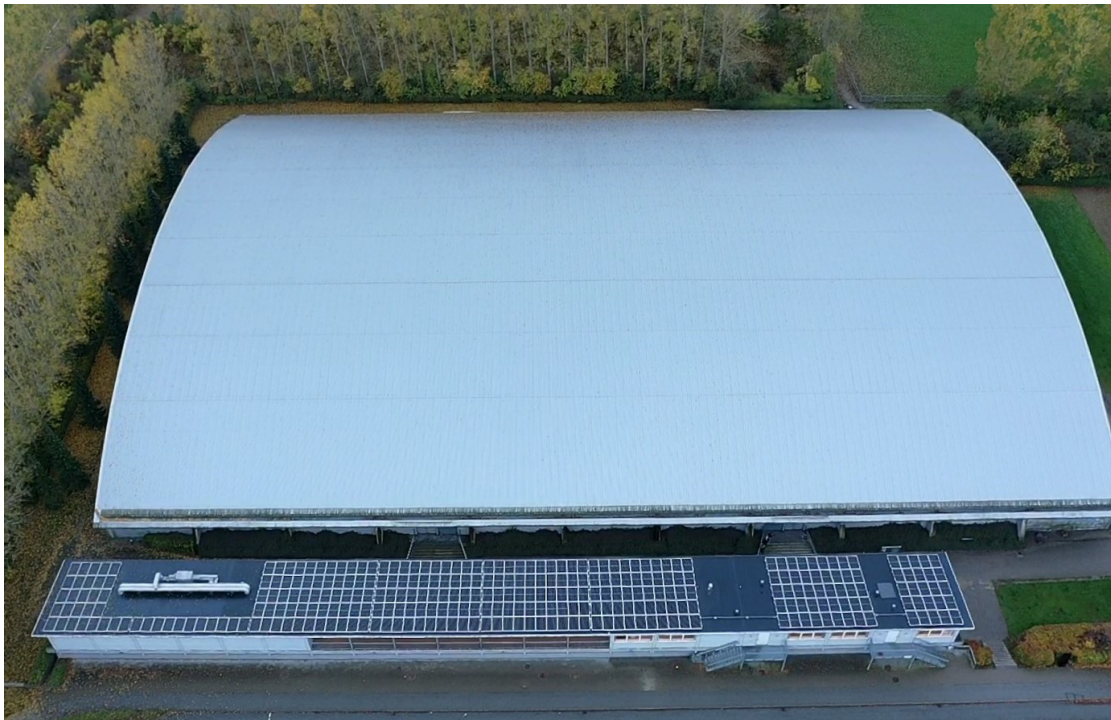
Fig. 1 The PV-system installed on the roof of the changing room building for TOPDanmark hallen.
