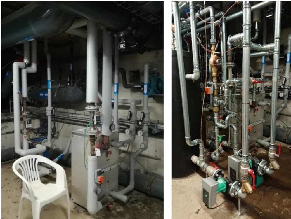
Fig. 3: Left photo: Heat exchangers for swimming pool (front) and hot water pool (rear) in the old installation. Right photo: New exchanger on the district heating supply and pipe installation for introducing heat from the heat pump.
