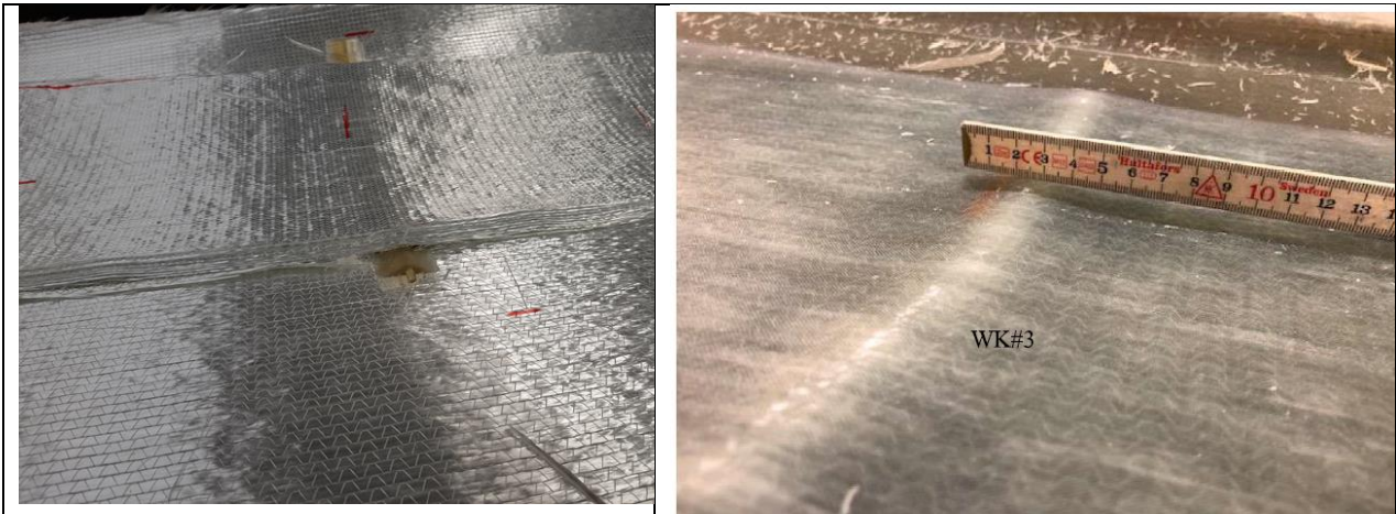
Figure 5.3.14. The picture to the left shows the placement of resin insert in between fiber fabrics and to the right a picture showing the wrinkle created by introducing the resin insert into the layup of pressure shell.
