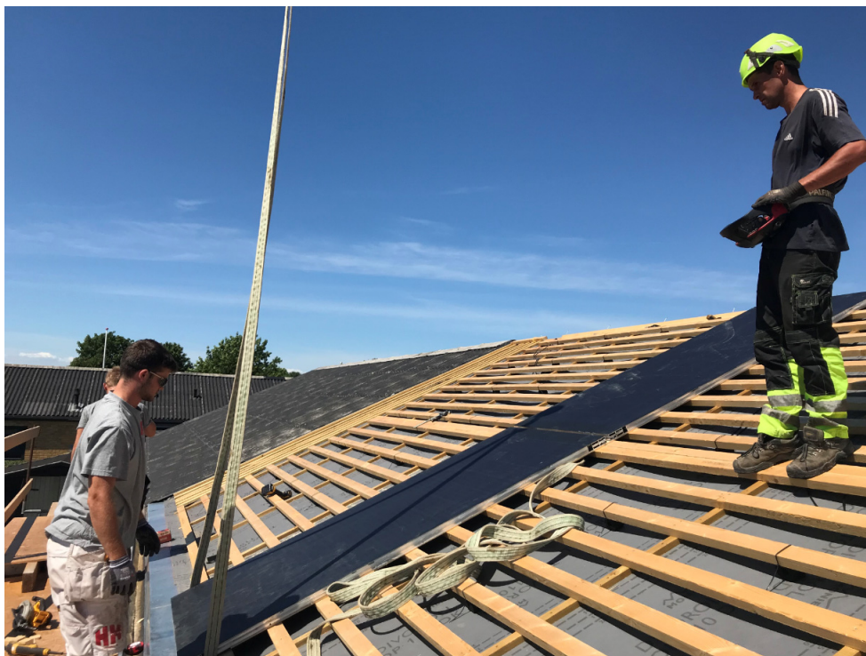
Large area modules being installed in the Stengården house in Ølstykke. Installation was done within 2 days only.
