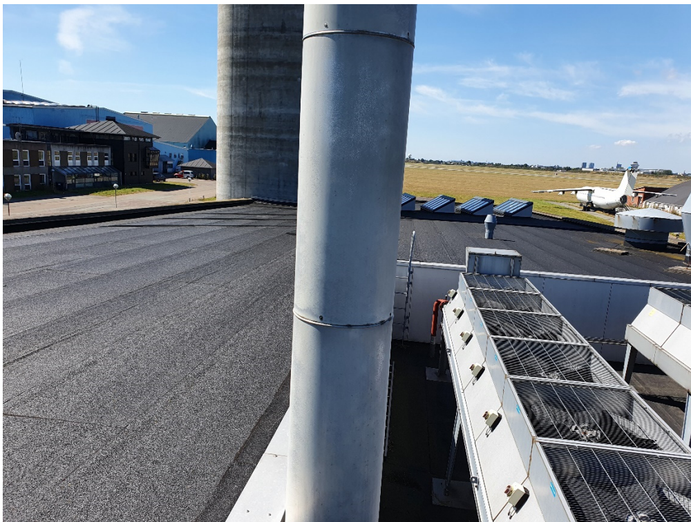
The existing air-cooling system to be replaced by the PVT-E roof Solar Smart System
