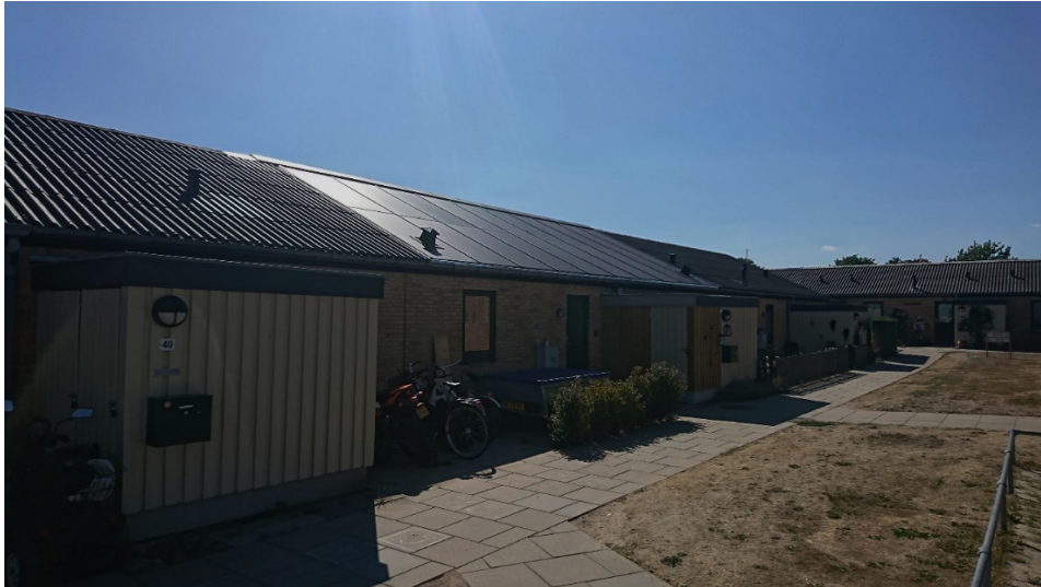
Figure 3.2.1 (I) The house chosen in Stengården at Ølstykke. Notice the two outlets. Holes were cut on site.
