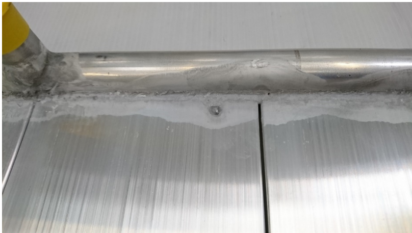
Figure 3.2.2 (III) The critical absorber with flame hand welded MPE profiles. Many failures occur during the hand welding and cause leakages afterwards. Leakage test is adopted, but the quality is questionable for surviving for more than 20 years. The aim is 50 years.
