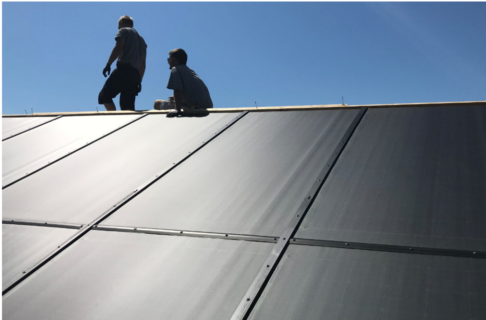
The PVT modules being installed as the new roof in the house in Ølstykke
