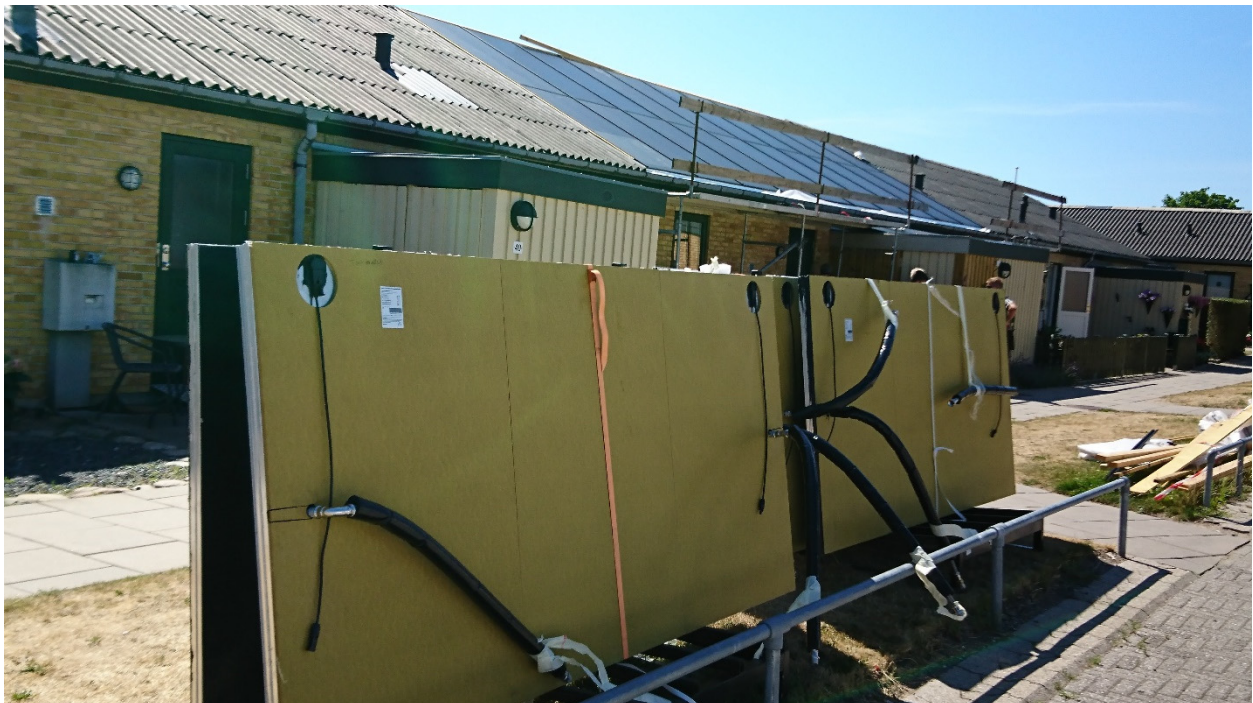
Figure 3.2.2 (I) Final PVT-E modules before mounting seen from the rear
