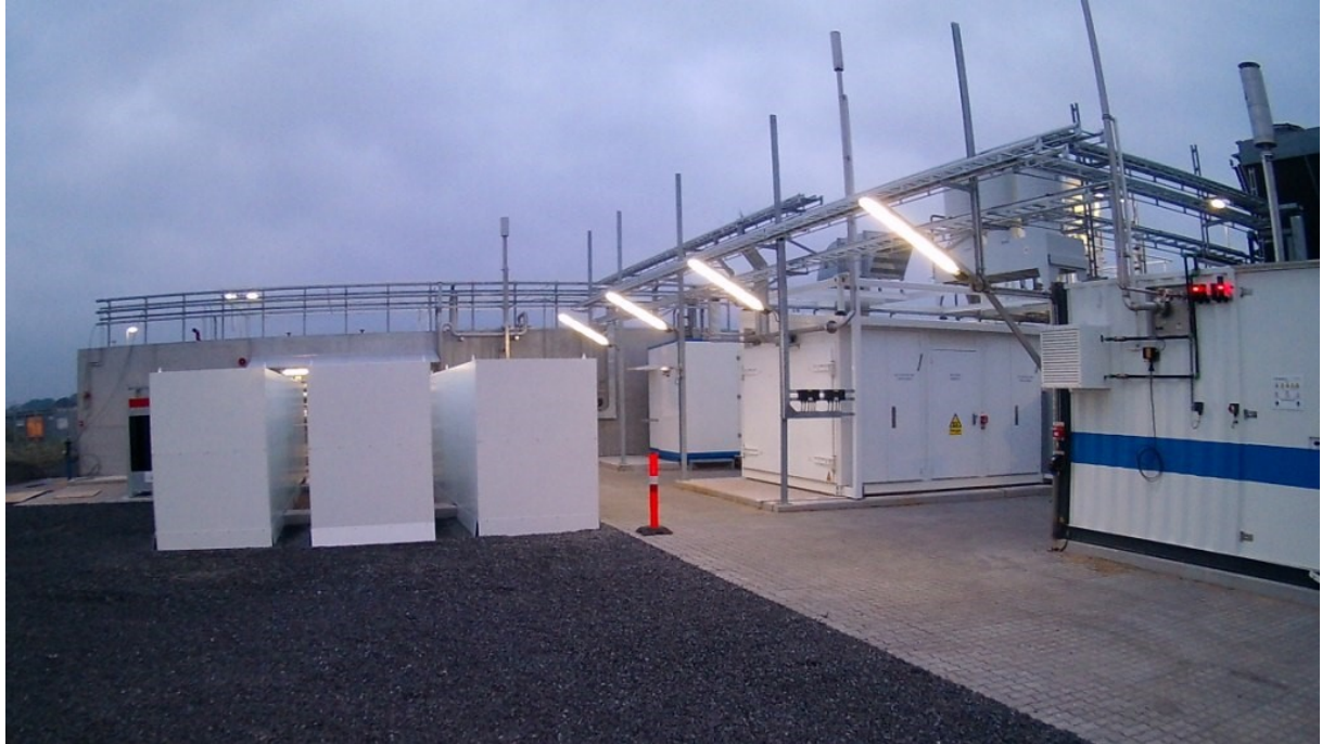
Figure 3 : Hybalance site connected to the main power
