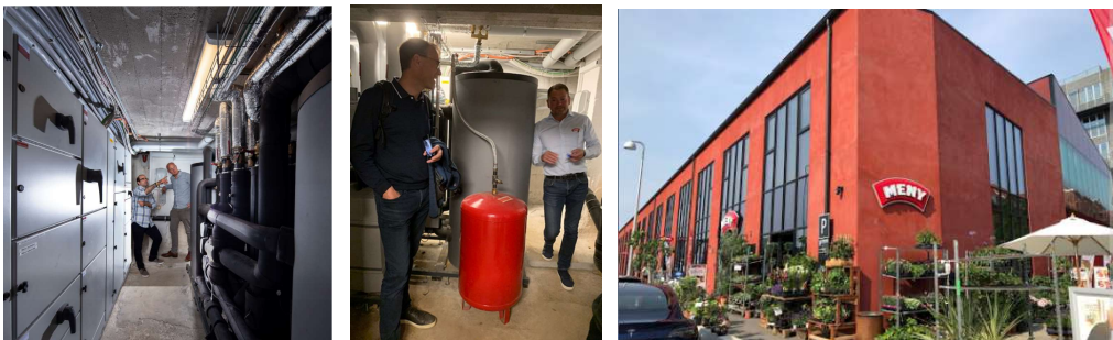
Figure 4 Pictures from the heat recovery system and the outer facade of the Meny supermarket in Nordhavn
