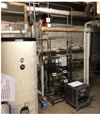
Figure 2. The circulation booster system installed at Strandboulevarden site.
