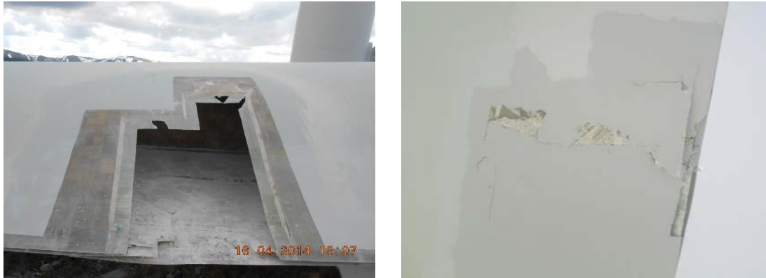
Figure 55: Extract of a blade inspection report showing transverse cracks in the max chord region on an infield wind turbine blade.
