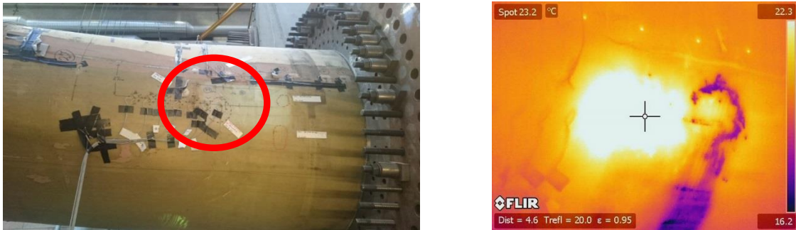
Figure 4: Left: Damage on the SSP34 blade, observed by visual inspection. Right: Thermographic photo of the same damage. The temperature at the damage location has been greatly increased.
