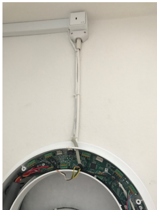
Figure 37. Installed BREATHE 55 unit in test apartment with Modbus cabling. The Modbus cable must be removed and reassembled by filter replacement, which is not appropriate optimal for a standard installation.
