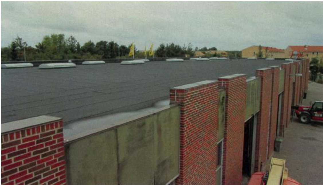
Visit a flat roof at Farum commercial Centre with focus on PV integration in 2012.
