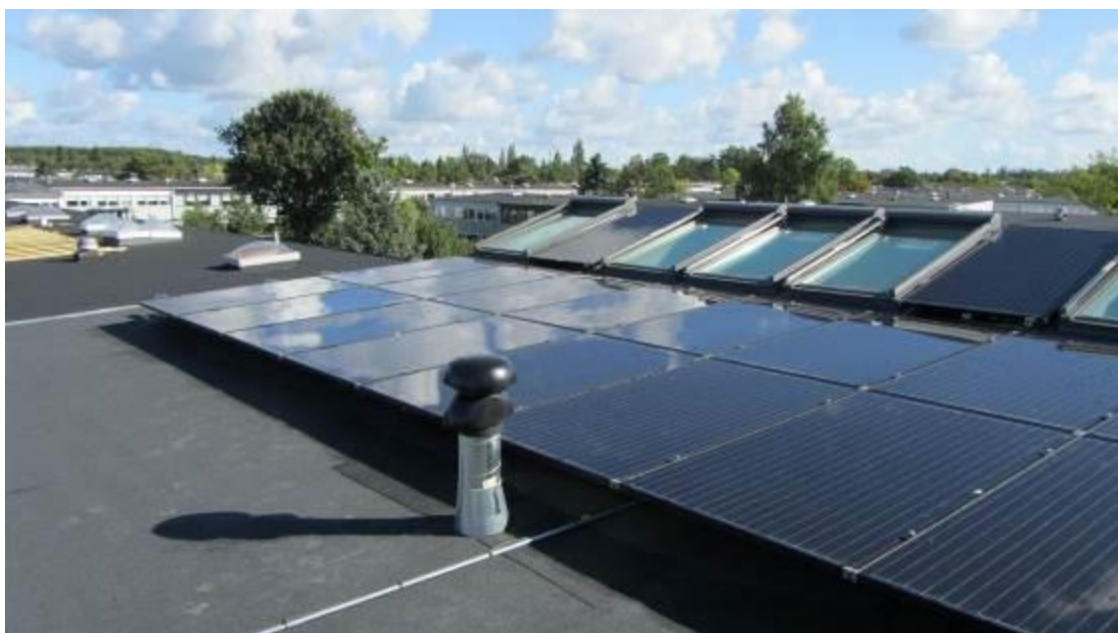
PV integration with VELUX windows at Albertslund.
