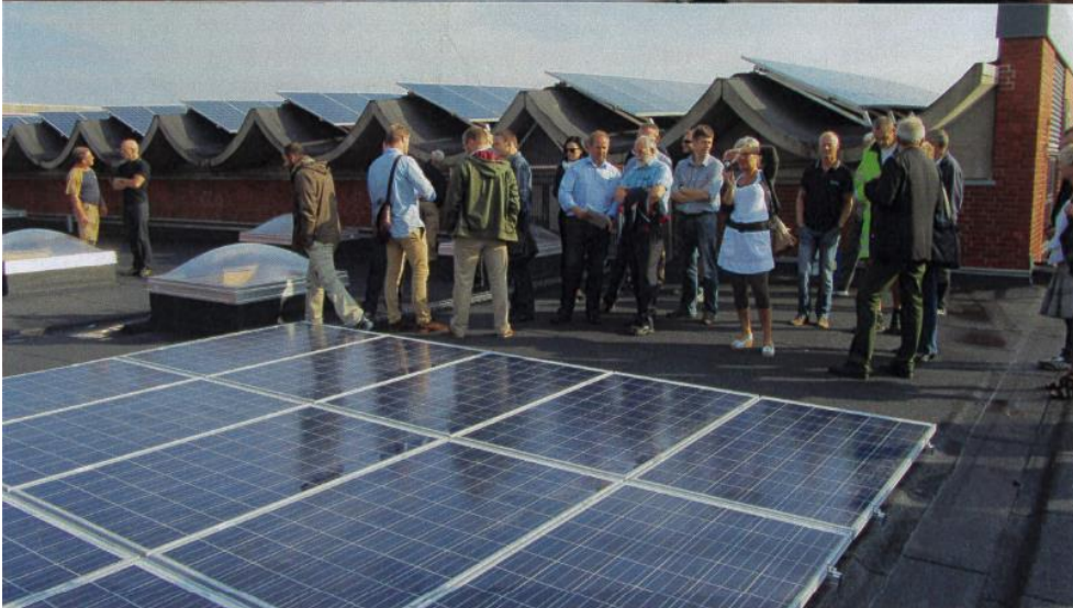
Illustrations from start up of 200 kWp PV installation at the Friheden Sports Centre in Hvidovre on basis of a sketch design project, design and tender made by Solarplan, Architect
