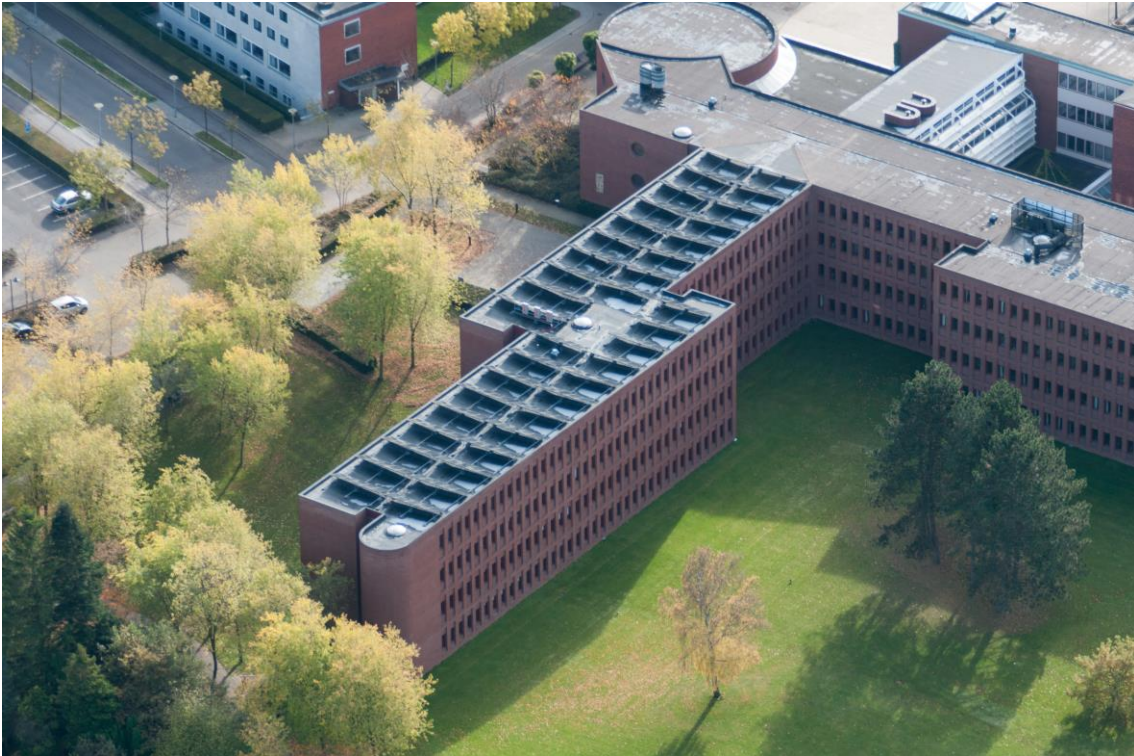
PV installed on Gladsaxe City Hall based on a PV-Cities sketch design project.
