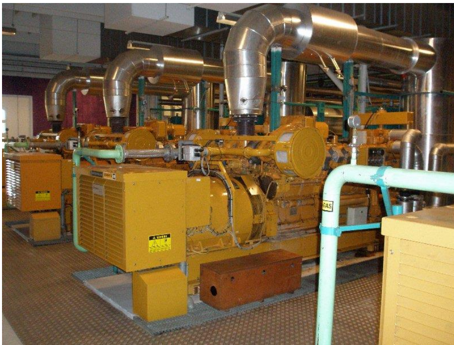
Figure 6 Gas engines at Dronninglund Fjernvarme
