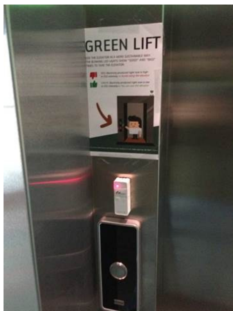
Figure 6 - Green Lift, blinking LEDs and posters were placed in the elevator to trigger behavioural change.
