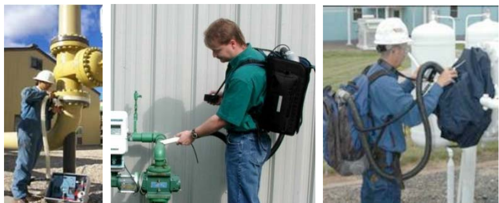
Figure 6 Example of a portable HiFlow Sampler for measuring leaking objects – in the picture to the right in combination with encapsulation of the leakage
