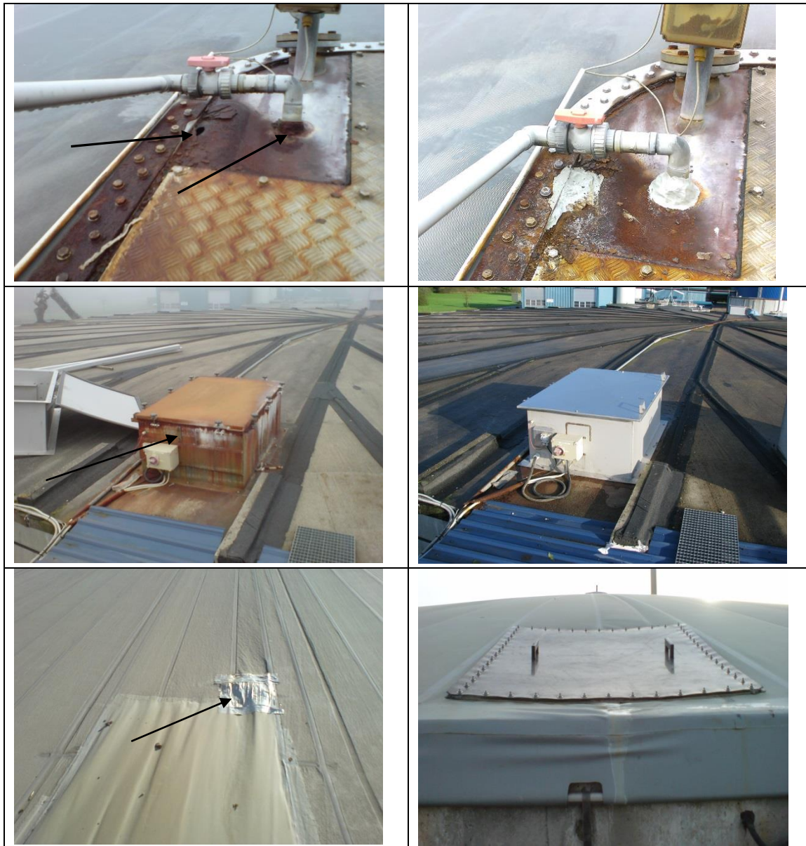
Figure 5. Examples of leakages repair. Top (left): Leakages identified at the cover of a digestate storage tank. Top (right): The identified leakages after being repaired with sealants. Middel (left): A leaking box covering a mixer situated on the roof of a covered digestate storage tank. Middel (right): The covering box was later replaced by a new box. Bottom (left): Leakage in a membrane covering a digestate stor- age tank. Bottom (right): The membrane was later replaced by a new membrane.
