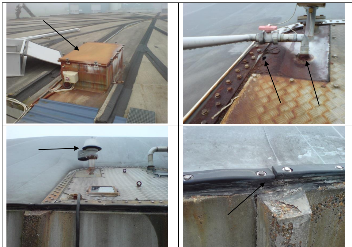
Figure 2. Examples of detected leaks. Top, left: Leakage through a box covering a mixer on the roof of a covered digestate storage tank. Top, right: Leakage through a hole in a covered digestate storage tank. Bottom, left: Leakage through a pressure safety valve. Bottom, right: Leakage through the assembly between the concrete wall and the membrane roof at a digestate storage tank.
