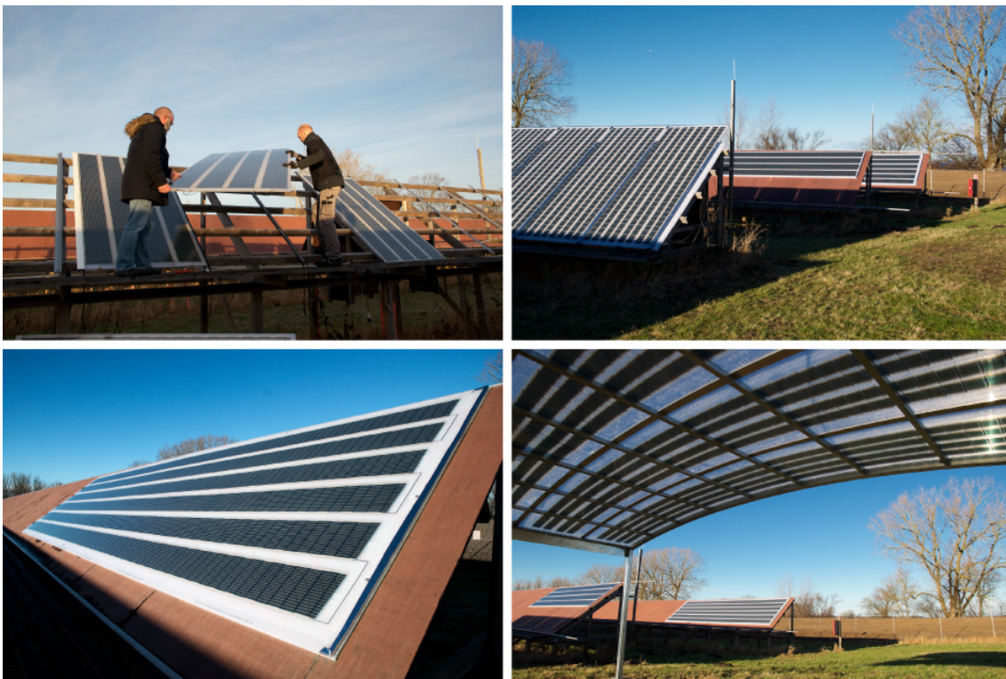
Fig 10 Various solar roof plate panels installed on wooden scaffolds and utilized as solar carport
