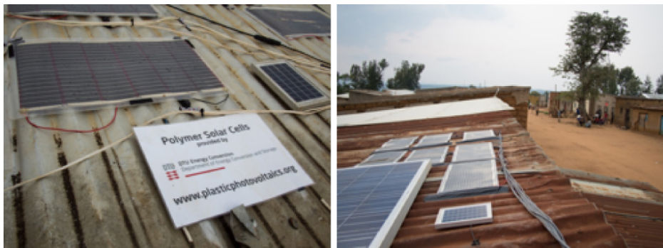
Fig 11. Polymer solar cell foils installed in Rwanda
