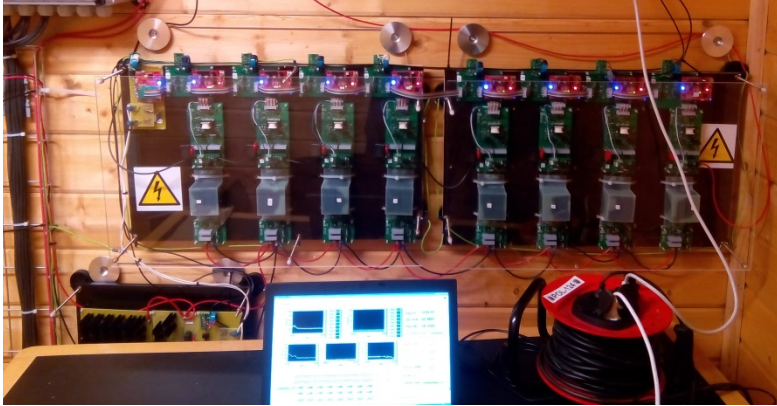
Fig 12. 8kV/1kV HV converter with eight stage and 2.4kW of nominal power.
