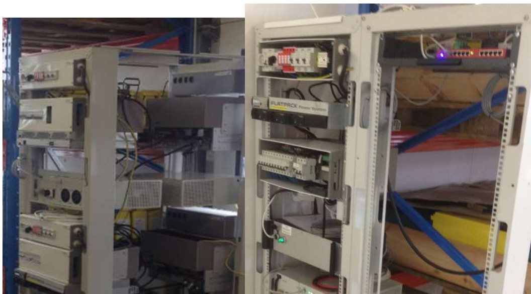
There are various charging systems at tele sites and different types of chargers are used.
