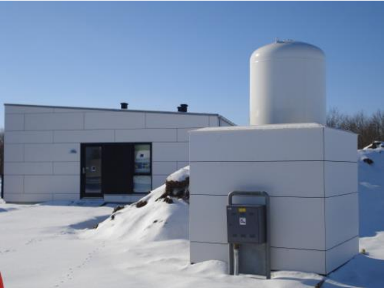
Image 1: Electrolyser building at H2 college
