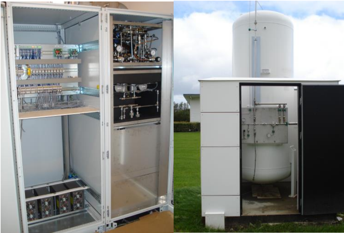
Image 2: Electrolyser system and storage tank
