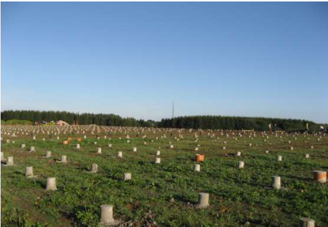
Fig. 6.12: Punctual foundation for solar collectors
