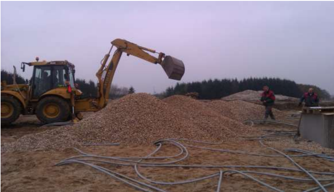
Fig. 6.6: Cockle shells and connection pipes
