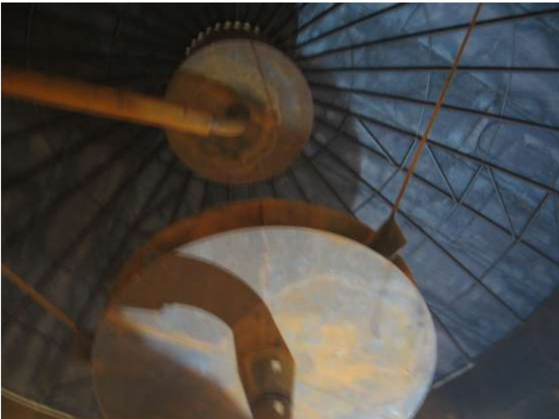
Fig. 6.11: In- and outlet in mid and top of accumulation tank
