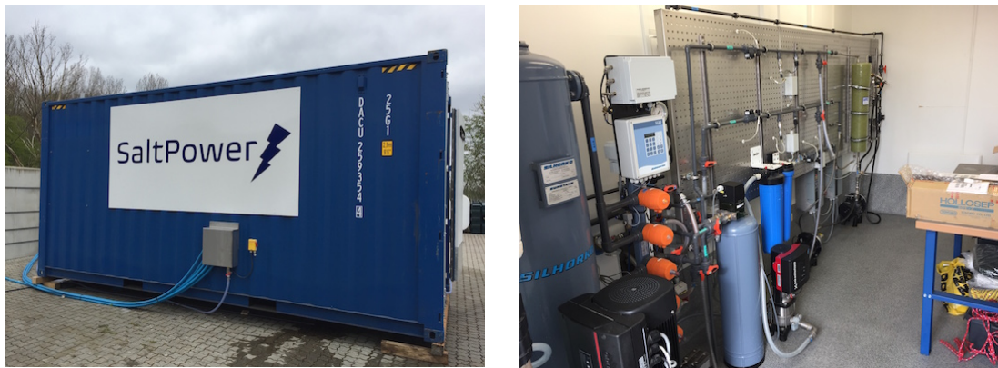
Figure 3 The finished pilot plant. To the left, the container can be seen with the in- and outlet manifold. In the background the reservoir tank can be seen. To the right, the interior of the container is shown. From left to right is seen: the sand filter, ion exchange softening, particle filtration, high pressure pump, osmotic membrane, and turbine.
