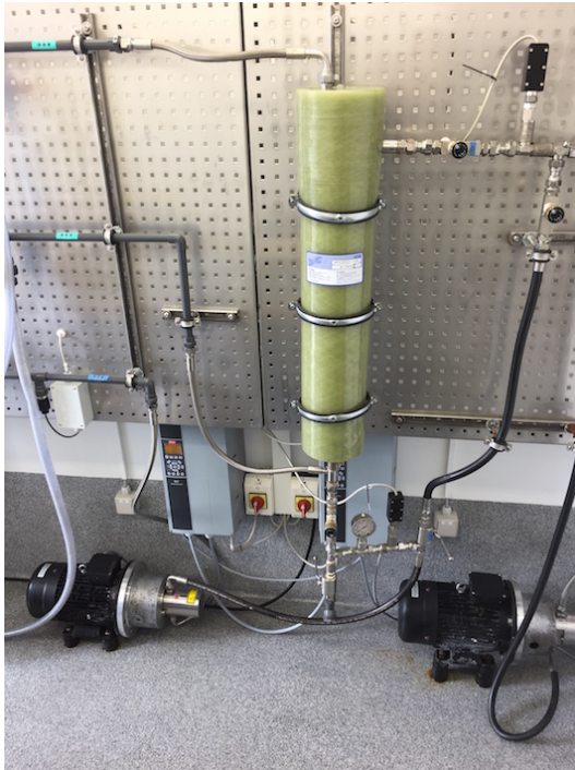
Figure 4 The heart of the SaltPower process. From left to right is seen: The high-pressure pump, the osmotic membrane and the turbine.
