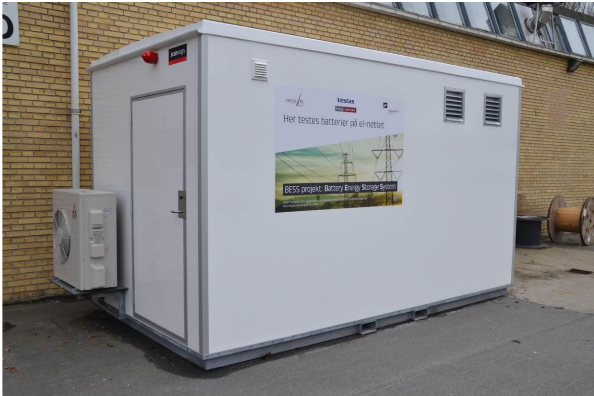
Figure 70: Picture of the installed Scale BESS system
