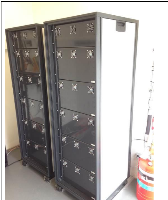
Figure 87: Picture of 1 battery string and control boxes installed in specialty House.
