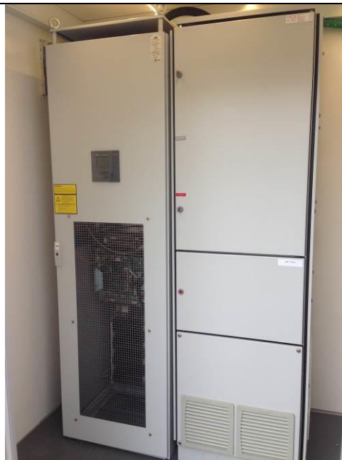
Figure 88: Picture of inverter and electric cubical incl. transformer installed in the specialty house.
