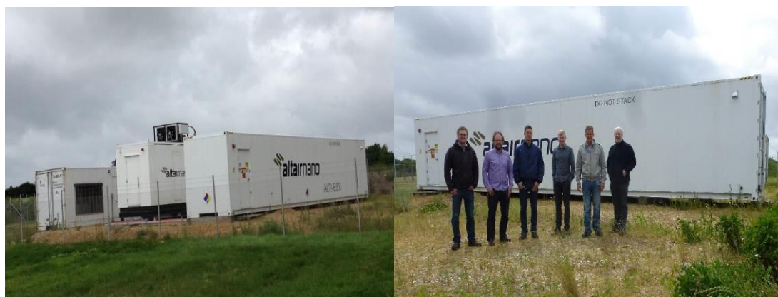
Pictures of BESS systems and the main project team in Lem Kaer
