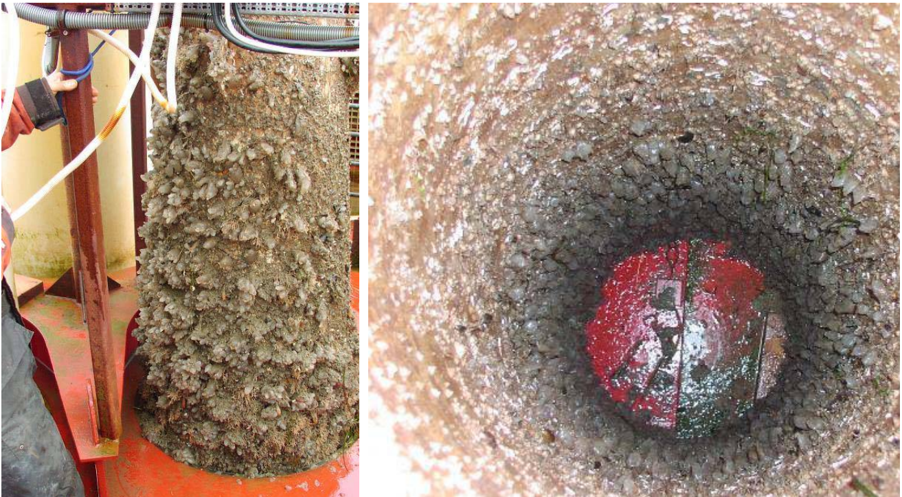
fig. 39: growth on epoxy painted draft tubes, outside and inside
