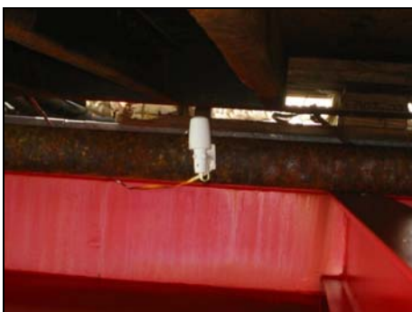
Fig. 2.5 Outdoor temperature & humidity sensor
