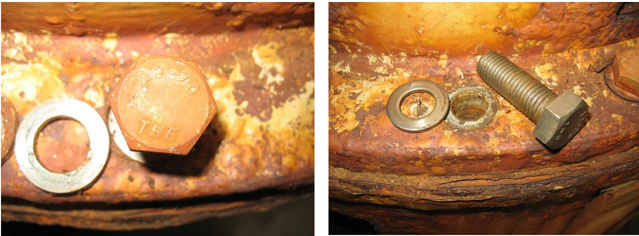
fig. 16: bolt connection of generator case and turbine shaft case
