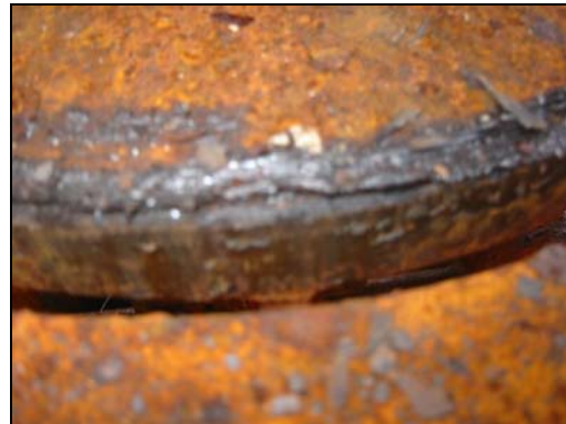
Fig. 3.7 Severe erosion of dummy turbine gate (11.08.03)
