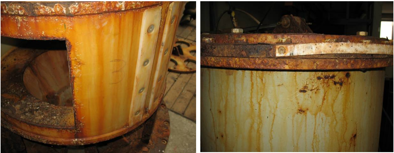
fig. 10: cylinder gate guide rails and bearing strips
