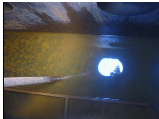
Fig. 5.14 Flooding of port shoulder
