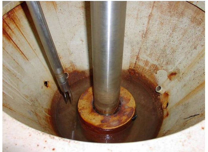
rubber bearing assembly turbine no. 5
