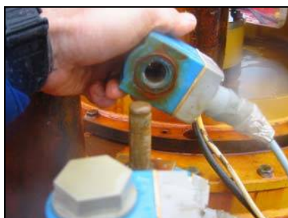
Fig. 3.5 Saltwater corrosion of solenoid (23.06.03)
