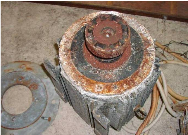
generator turbine no. 7
