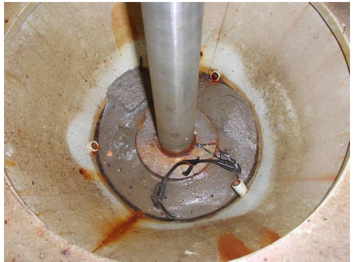
rubber bearing assembly turbine no. 3
