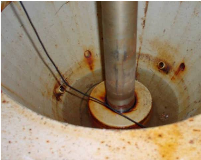
rubber bearing assembly turbine no. 4
