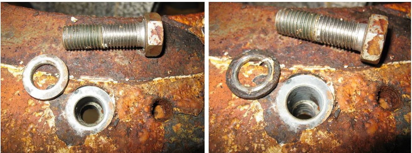
fig. 15: bolt connection of upper generator deck
