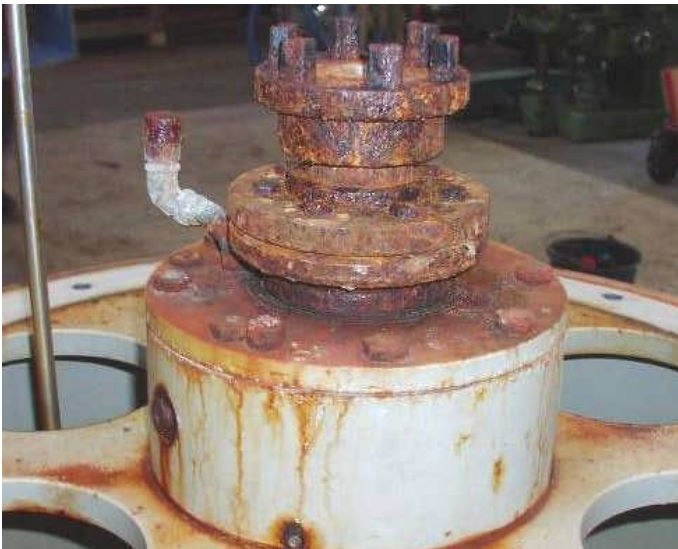
thrust bearing assembly turbine no. 3
