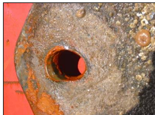
Fig. 5.24 Original damage caused by fishtail plate bolt
