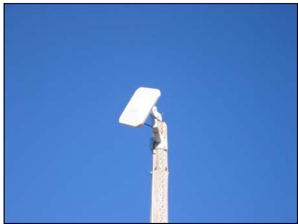
Fig. 8.2 Wooden pole with transmitter attached
