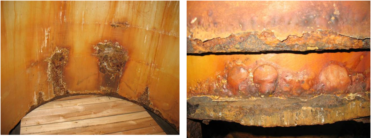
fig. 8: cylinder gate – corrosion on lower edge
