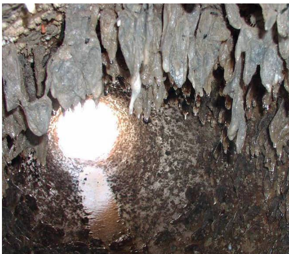
draft tube with conventional epoxy paint
