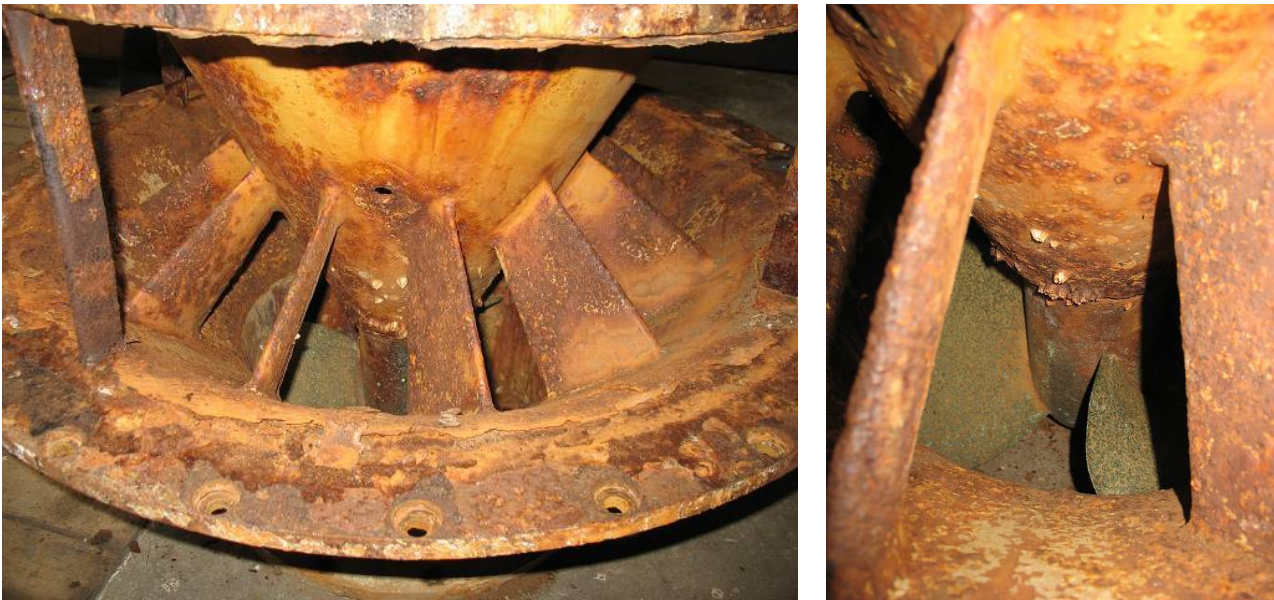
fig. 32: inside of bearing shell and radial bearing section of the turbine runner shaft
