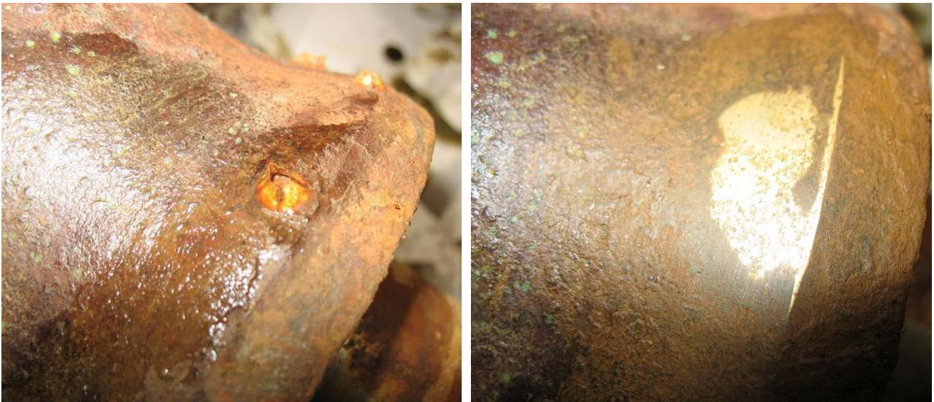
fig. 36: corrosion on turbine runner
