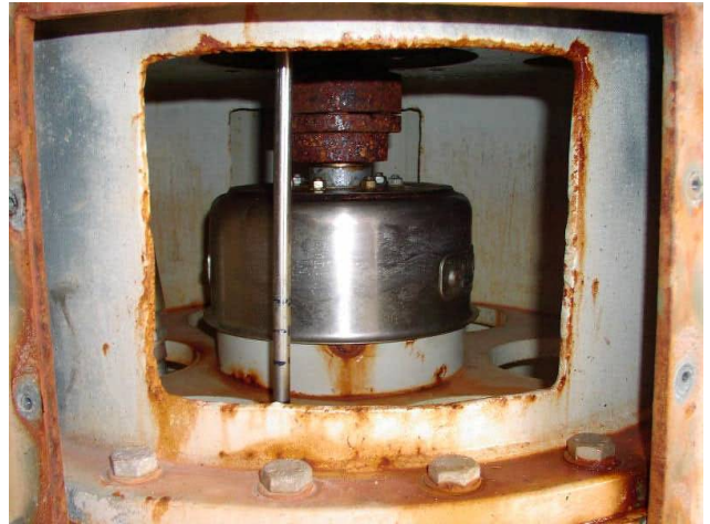
thrust bearing assembly turbine no. 5
