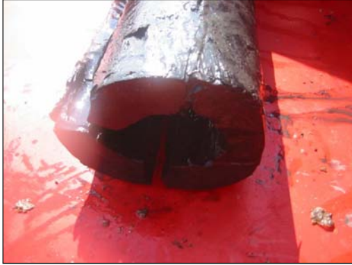
Fig. 5.19 Rubber fender damage
