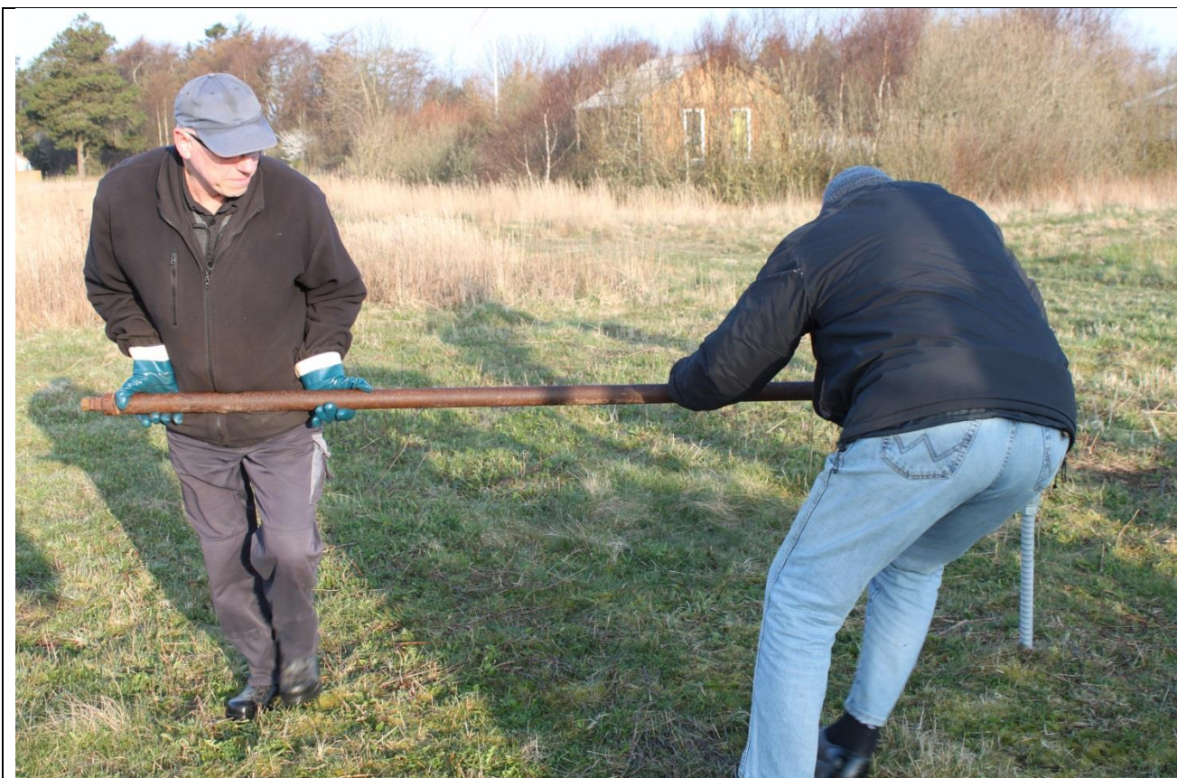
Torque applied to drive the anchor 2 m into the ground: 40 \text{ kg} \times 3 \text{ m} = 1200 \text{ Nm}
