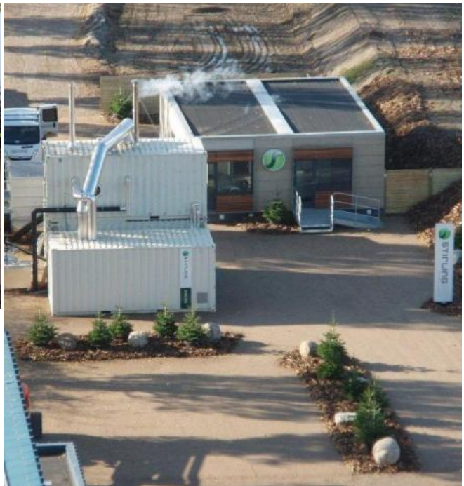
Picture 8: The Stirling engine plant in operation with the visitor's centre behind it.
