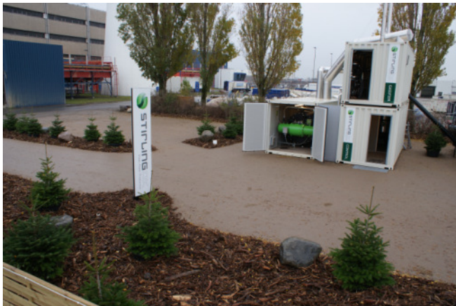
Picture 7: The Stirling engine plant at Amagerforbrændingen.
