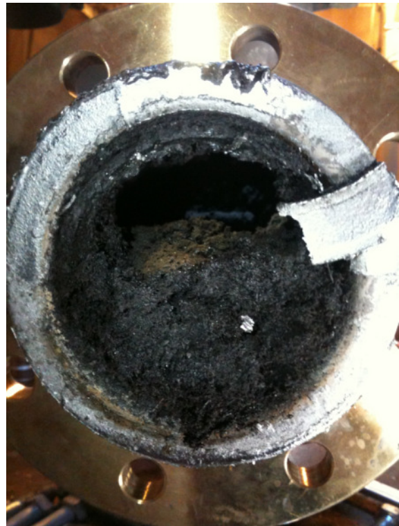
Picture 16: Blocked product gas pipe after willow chips test run
