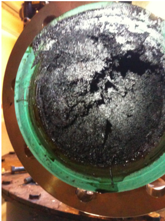
Picture 15: Blocked product gas pipe after willow chips test run
