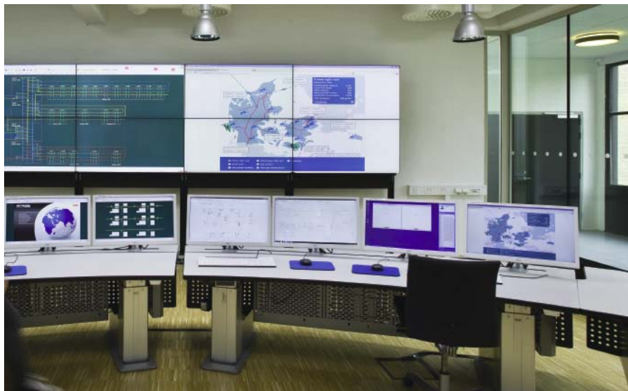
Figure 2-9 : A full scale SCADA system, ICL
