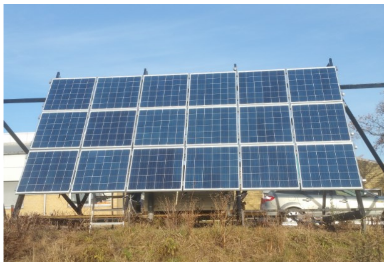
Figure 23: Outdoor testbed for I-V and IS measurements with 10 measurement channels.
