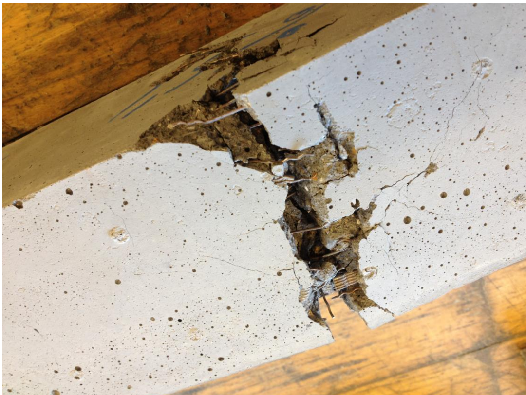
Figure 8 Failure surface of beam where bundling of the long fibres is visible.
