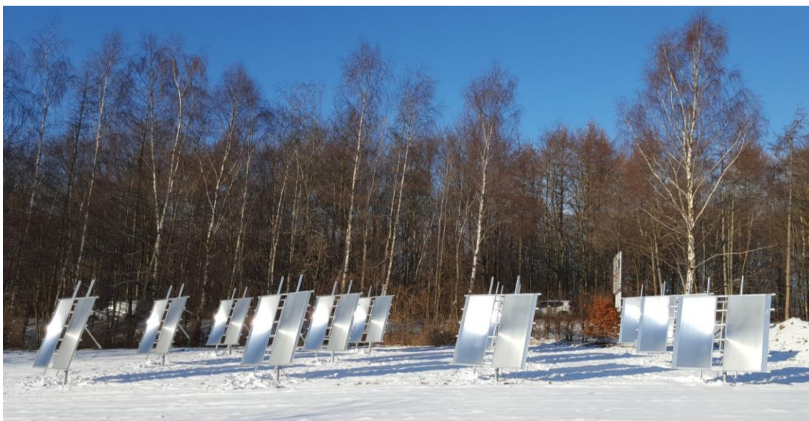
First 12-unit plant (before mounting of receivers)
