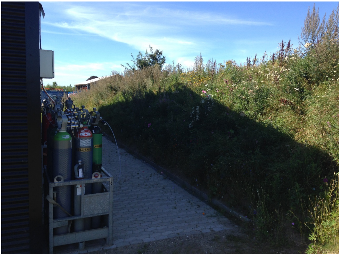
Figure 3: Top: The gas source for the laboratory, placed outside. Bottom: Safety has been of great concern in the design of the laboratory, all in compliance with the local fire department. Especially the rampart, securing the neighbours, was considered a great addition.
