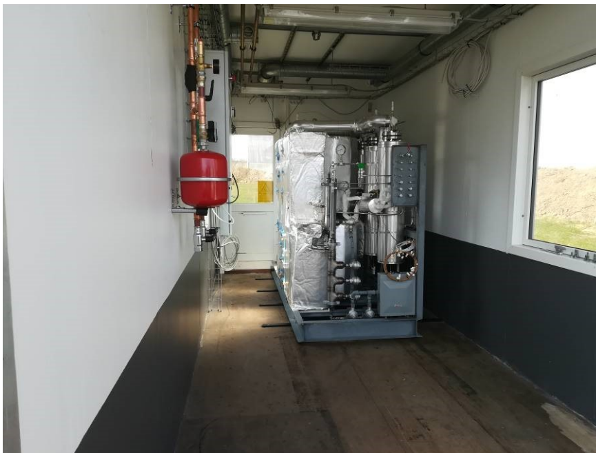
Figure 9: The picture shows the methanisation unit just after it was moved into the container. Following this step, the electric control cabinets, gas control cabinets, ATEX biogas compressor, biogas cleaning plant, gas analysers etc. were installed. The reactor was placed on four rails. This ensured that it was possible to do service on both sides, if necessary. During normal operation the reactor is placed close to the wall to the right.
