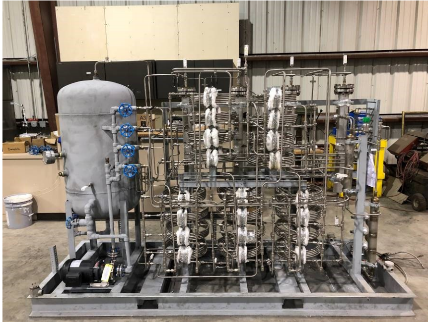
Figure 8: The picture shows the methanisation unit before all the parts were insulated. To the left there is an oil tank and pump below for the cooling oil that operates at temperatures between 200°C and up to 400°C. The coils are tube heat exchangers.
