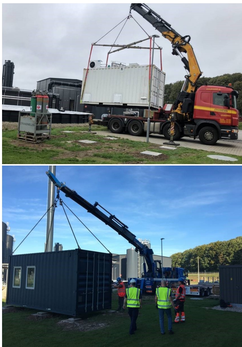
Figure 2. Moving the containers with the electrolyser (white) and cleaning plant and the methanisator (blue) to Midtfyn Biogas in late September 2018.
