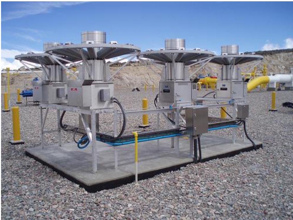
Figure 8 Gentherm power supply used e.g. for telecom radio link repeaters at remote locations, e.g. mountain tops, without access to the power grid. The photo shows a 2 kW system with four units each generating 500 W electrical power.
