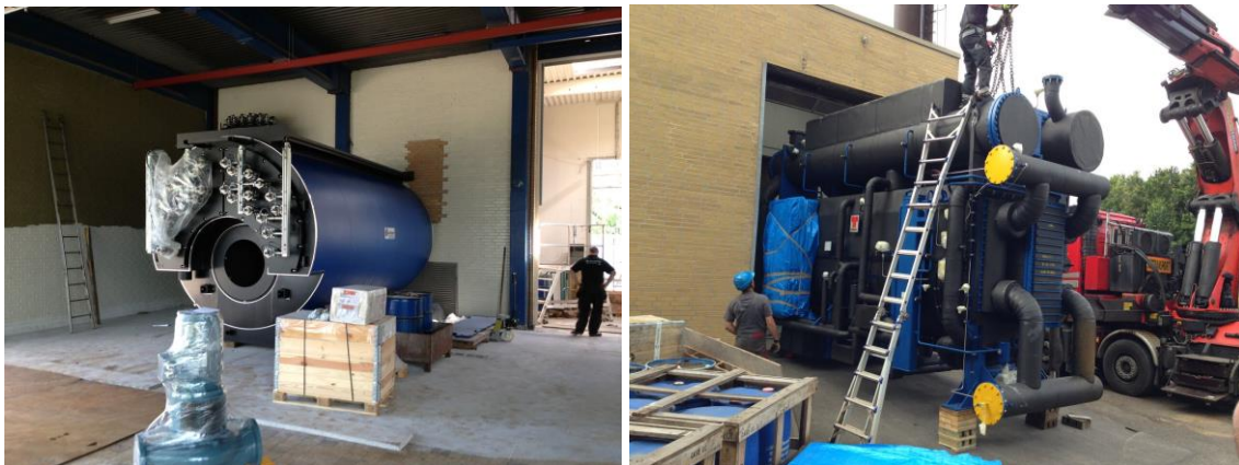
Fig. 14: Pictures from implementation in Søndervang (Boiler for absorption heat pump and absorption heat pump).
