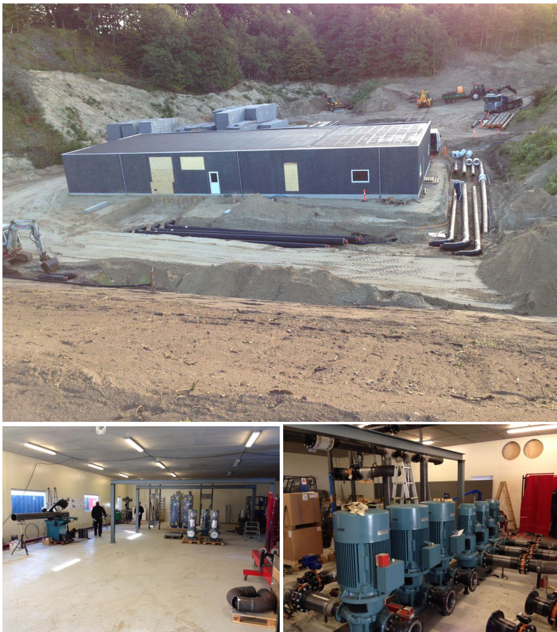
Fig. 15: Pictures from implementation in Lunderbjerg (Building, heat exchangers and pumps).
