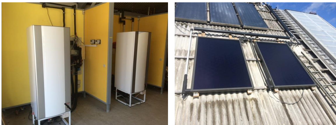
Figure 8 Pictures of the storage tanks and solar collectors in the two SDHW systems.
