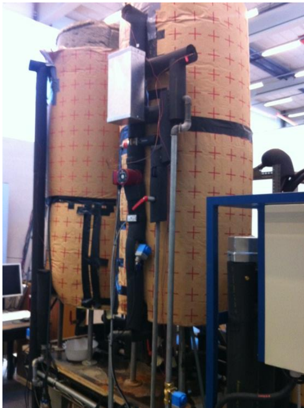
Figure 12 Photo of the two tanks and the test facility. Hot water tank (left) and hot waterstore (right).
