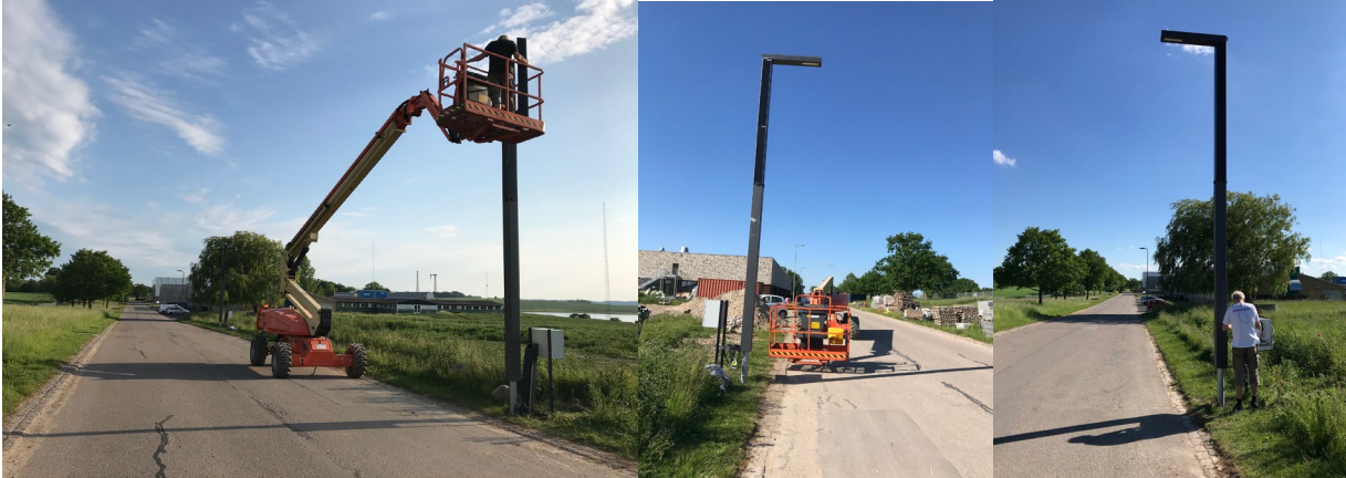
Figure 39 – SolarDesign lamps installed on Risø Campus for field test.
