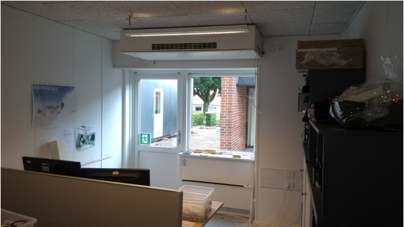
Figure 2: AMHVAC prototype installed at field test (office in temporary modular building, Rønde Efterskole).
