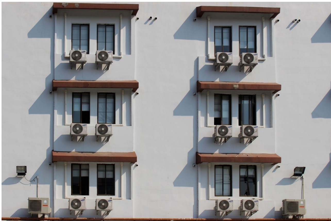
Figure 1: The well-known architectural problem and installation challenge we solve in this project.
