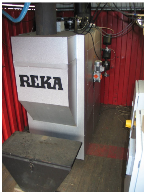
Figure 6. ESP for batch fired straw boiler. The filter is with a system for heating-up the insulators prior to start of the combustion and flue gas purification.
