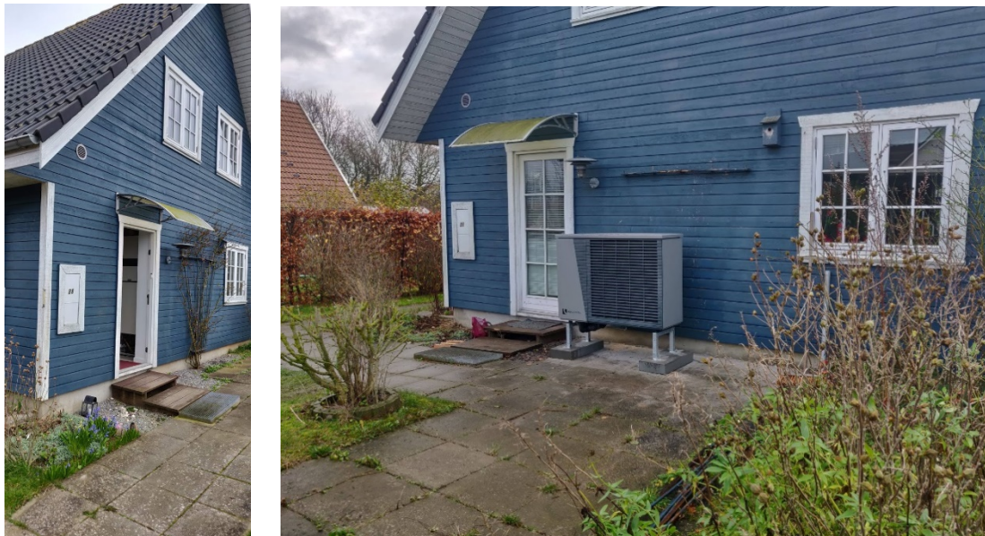
One of the field test houses in Lolland, before and after installation
