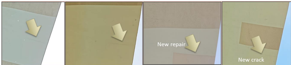
Figure 31: Showing development of crack after previous crack was repaired.
