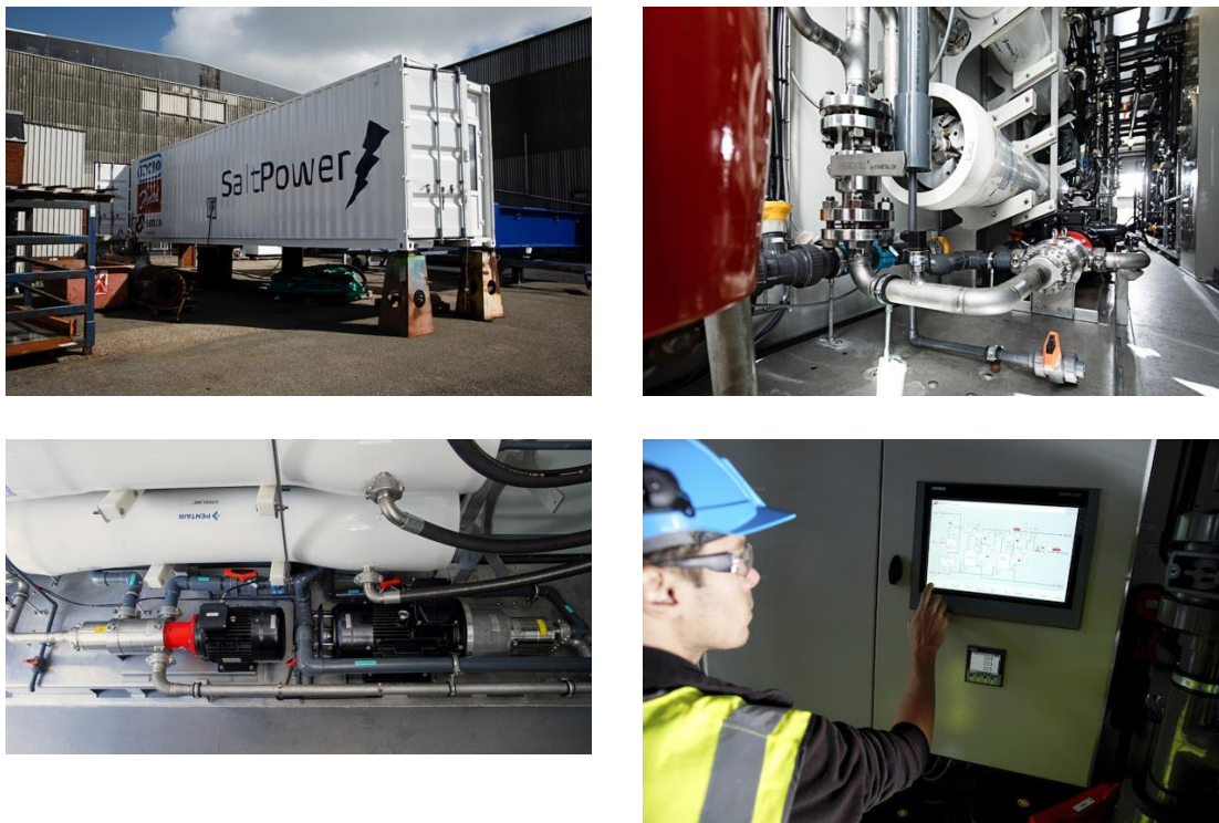
Figure 1: Photos of the demonstration system
