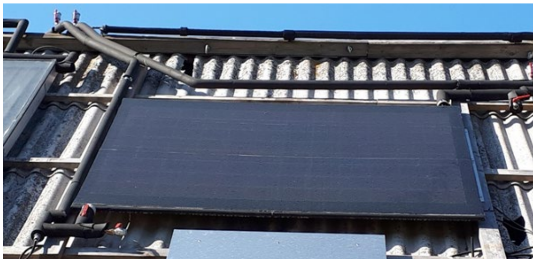
Figure 1. PVT panel installed at roof facing south with a tilt angle of 45°.
