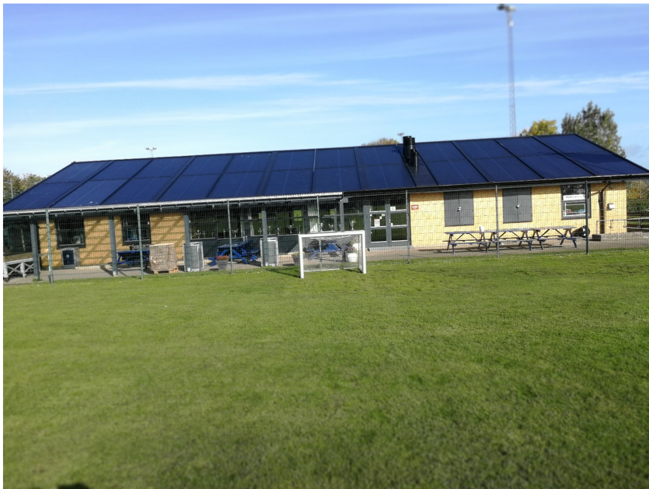
Figure 33. View of the PVT system integrated in the roof of the football club house in Stenløse.
