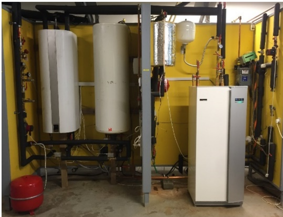
Figure 2. DHW and cold storage tanks and heat pump in indoor test facility.
