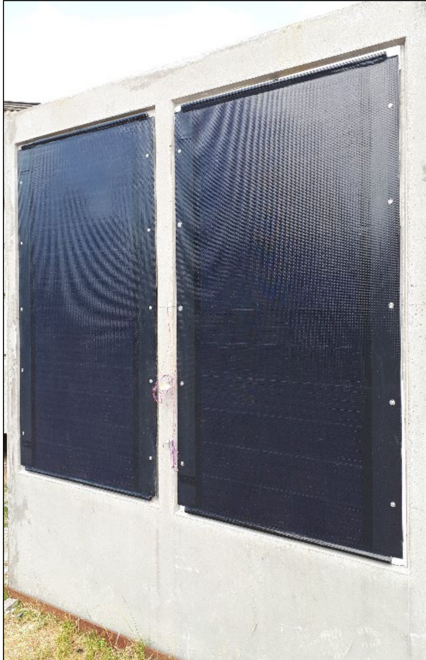
Figure 21. PVT panels integrated into a concrete facade.
