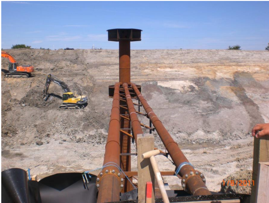
Figure 11. In-/outlet arrangement led through the side of the storage. Photo from the implementation of the SUNSTORE 4 storage in Marstal.
