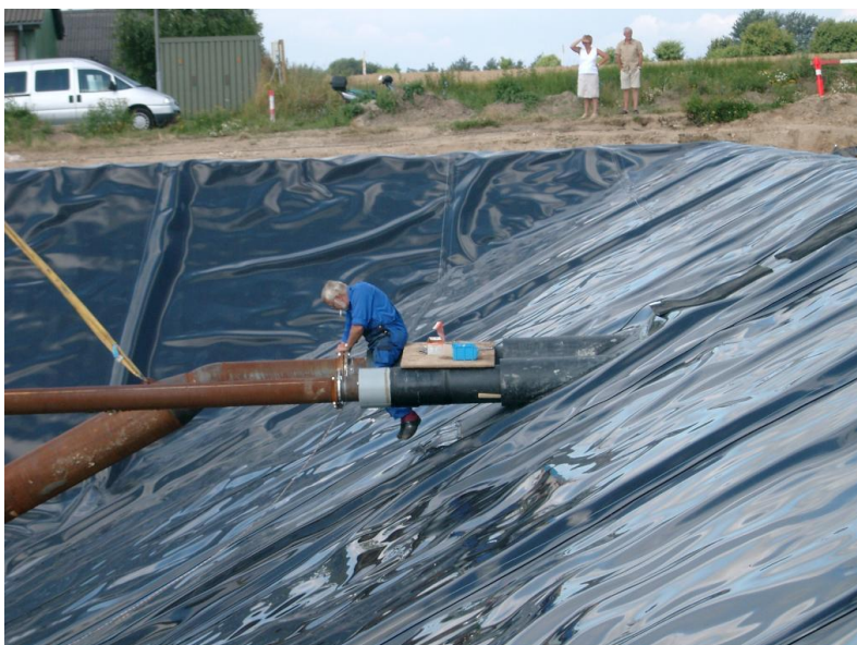
Figure 17 Inlet and outlet pipes. The leak was in the liner weld during one of the pipes [10].
