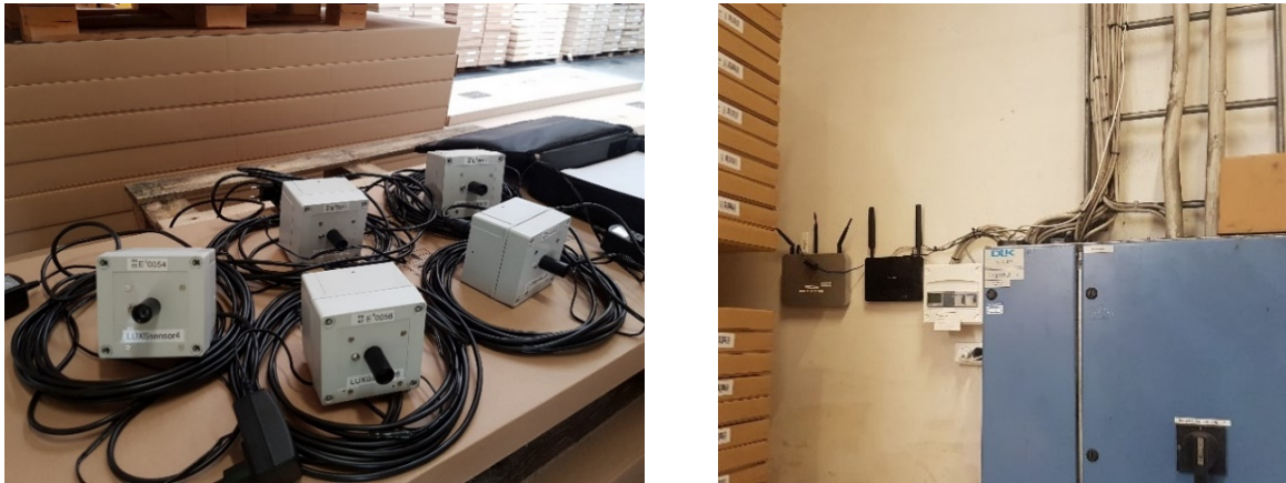
Figure 7. Photos from installation hall, left: five of the LuxSensors with long wires to be hung from the ceiling, right: routers for communication and installation of power measurement.
