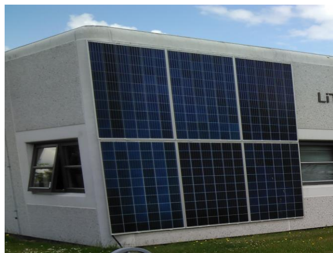
Picture showing the PV array used in the test
