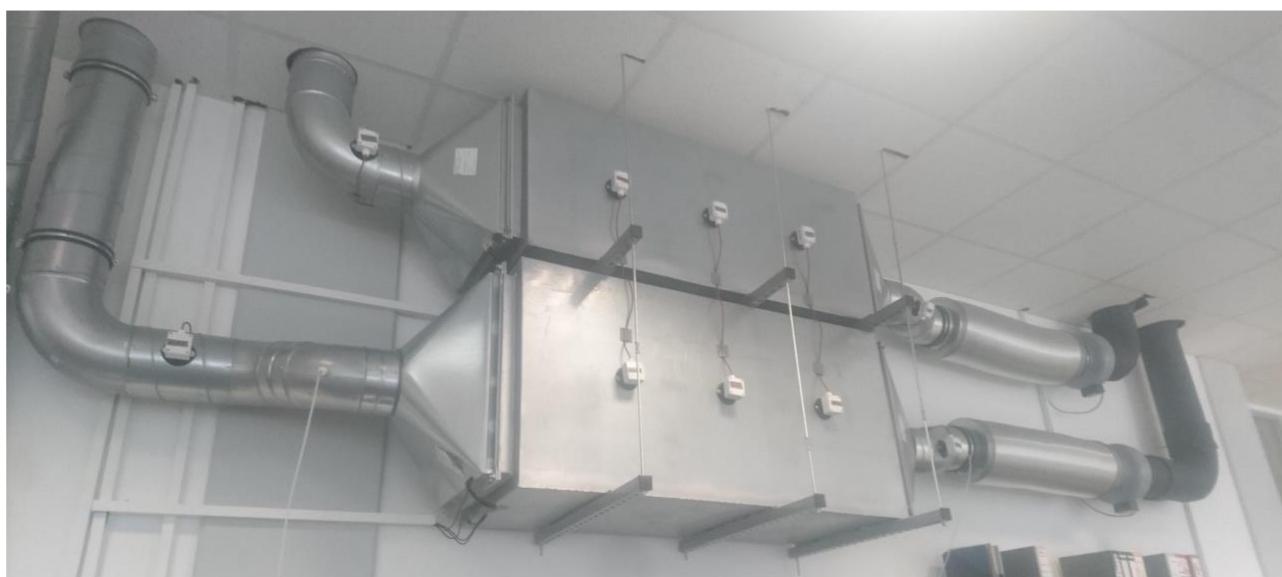
Figure 3. The actual PCM-driven ventilation system running at the premises of project partner Rubitherm in Berlin
