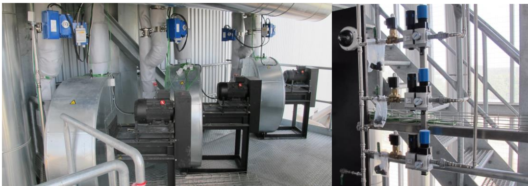
Figure 6: Left: The three hot air fans, distribution dampers, etc. Right: Emergency cooling systems and camera.
