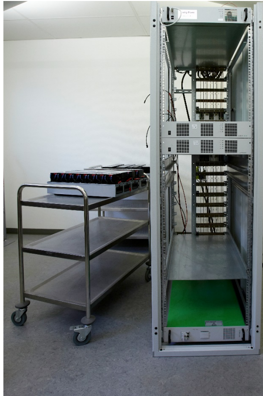
Figure 5.2. The power subsystem in laboratory testing. The unit is equipped with two power modules (mid position) and a battery management module (bottom position). A single battery string is used (left to the unit), offering 5.4 kWh storage.
