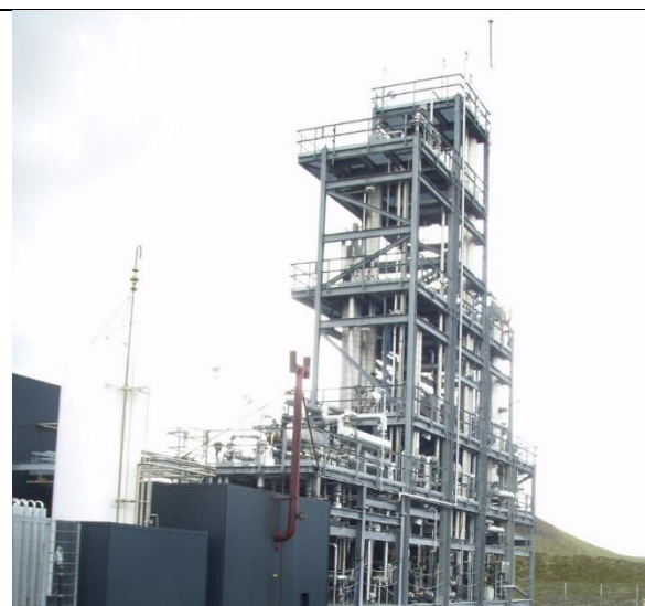
Figure 32 Power-to-Liquid, George Olah Plant in Svartsengi, near Grindavik, Iceland, 2012. Capacity 5 mio. liters per year.
