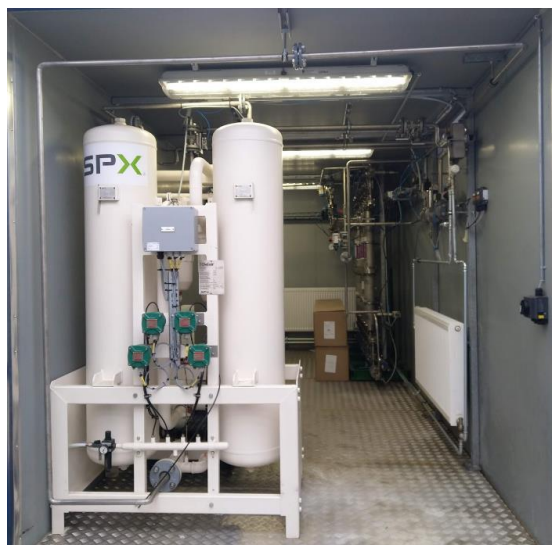
Figure 8. Containerized gas post-processing unit.
