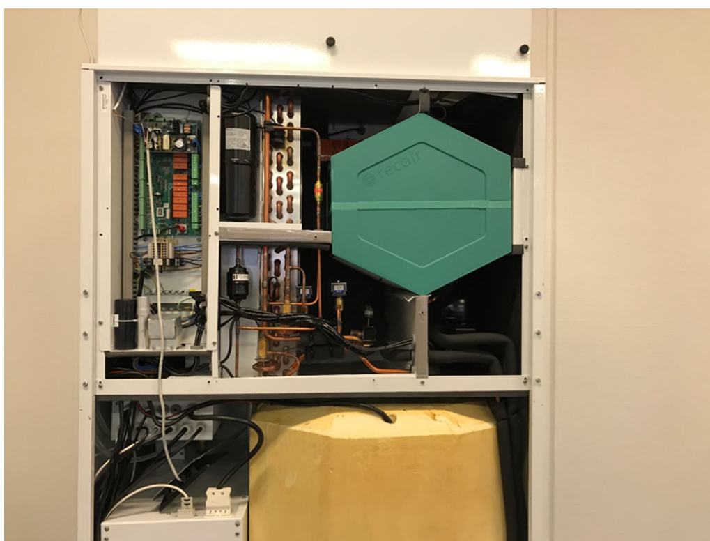
Figure 2: A look inside the existing Nilan ventilation heat pump.
