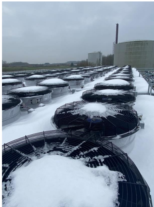
Ice and snow on top of the evaporators
