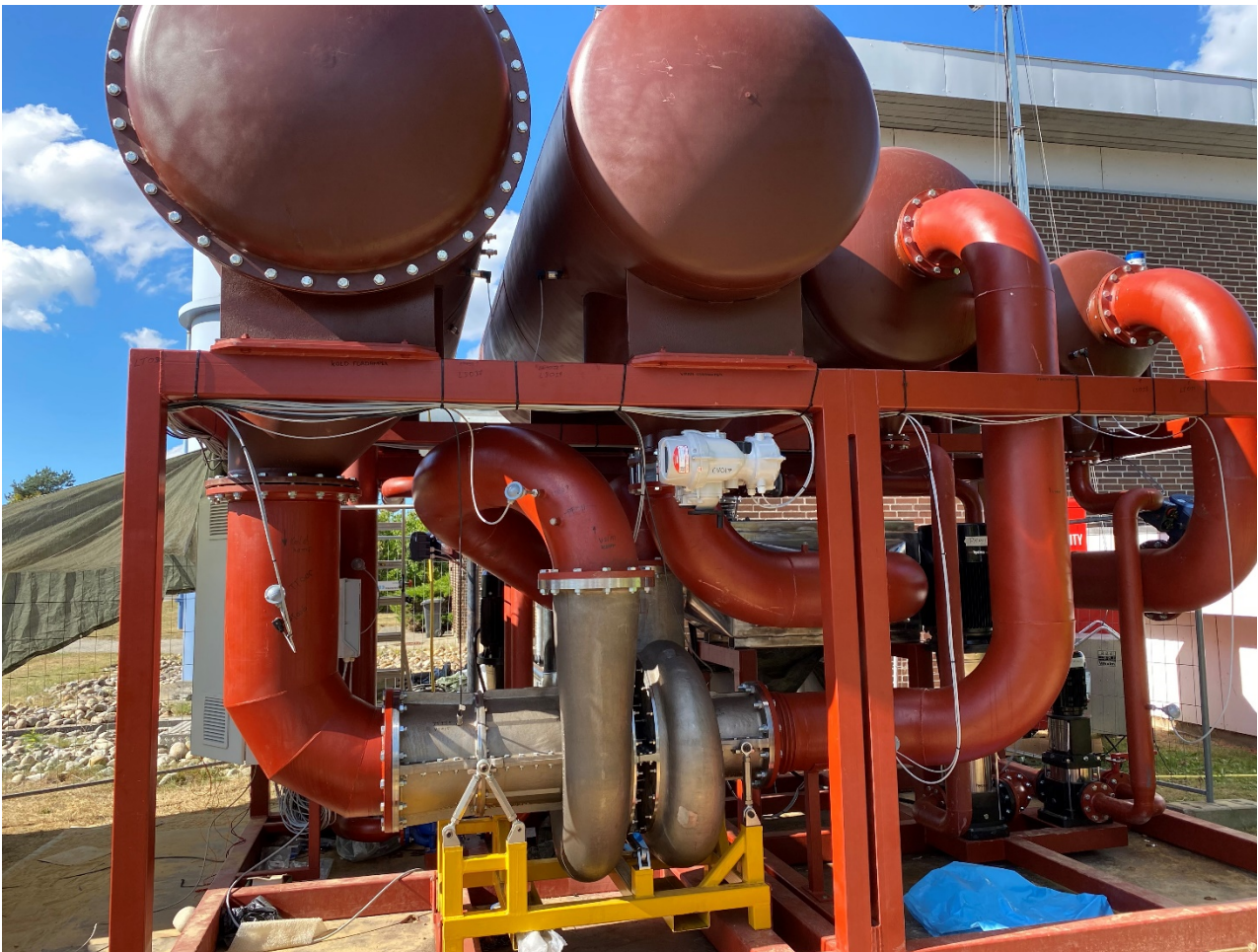
Figure 17 (same as figure 1): The STAC Technology chiller pilot has been assembled and installed at the test site. A constant water through put has been achieved. This has been accomplished using the automation setup developed to monitor and control the many valves and water pumps. The chiller has been pressure tested and the desired vacuum levels has been accomplished. Steam has been produced in the hot cycle to spin the turbine.
