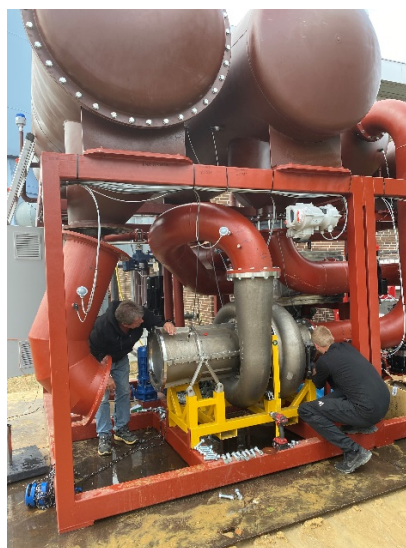
Figure 84 Detail on test plant assembly
