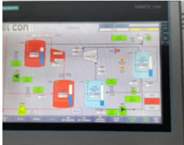
Figure 18 The chiller is fully automated and may be controlled by this touch screen interface. The outline of the sensors, actuators etc has been uniquely developed for this project.
