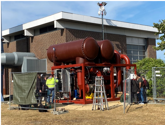
Figure 12 Test plant at Varde District heating
