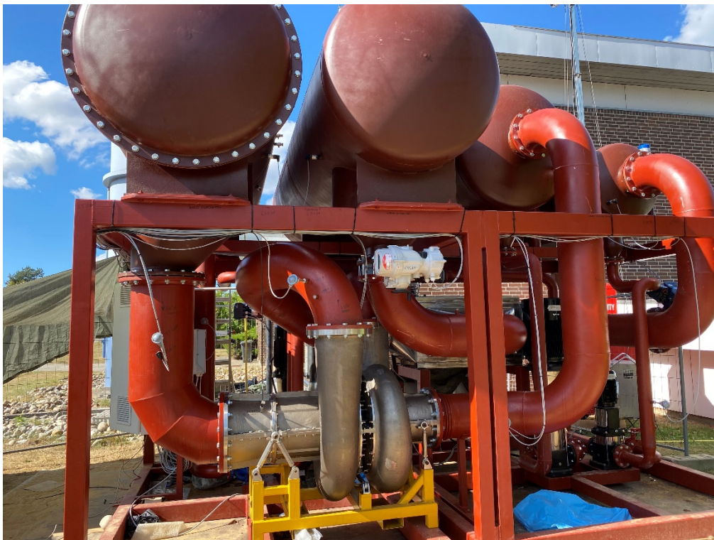
Figure 1 - 250 kW cooling plant placed at Varde district heating
