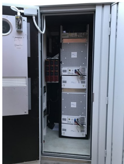
Figure 2 - Technical room Power shelter
