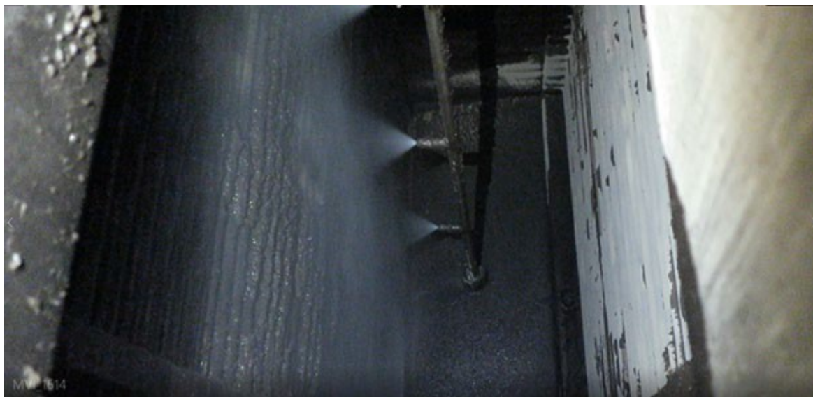
Figure 2 Picture of the water injection system installed in the LUFO (look through an inspection port). A lance with three nozzles is spraying water on heating tubes inside the LUFO.
