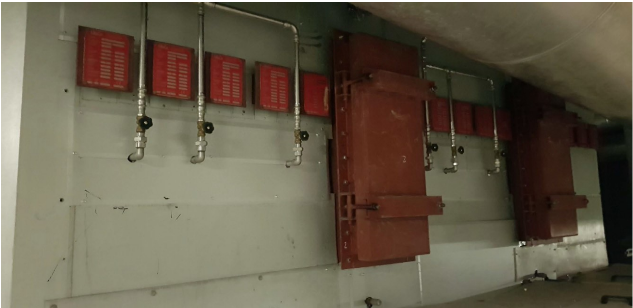
Figure 1 Picture of the water injection system installed in the LUFO (right hand side). Black valves for 6 of the lances with nozzles can be seen on pipes on the side of the LUFO.
